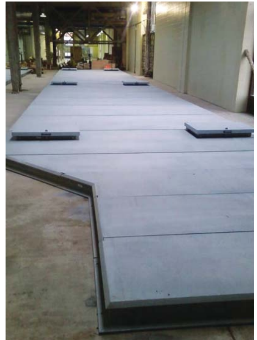
XL6 clear span tank cover system with angle cut panels and access hatches over filtrate storage tanks
