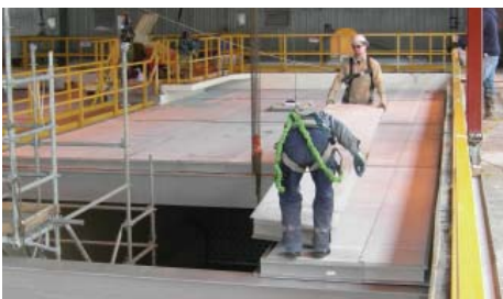
XL6 beam-supported cover - DAF cells. Cover panels can be handled by 2 workers alone.
