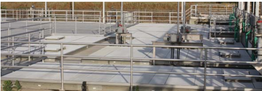
XL6 clear span tank cover system with access hatches UV Disinfection Process
