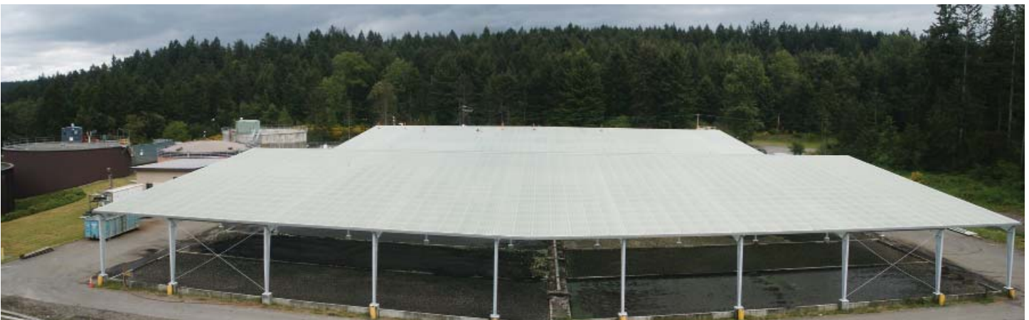
Tuff Span roof cover system Sludge Drying Bed
