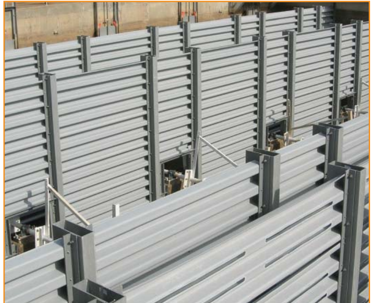
"D" structural baffle wall system - solid and slotted with FRP columns Sedimentation and Flocculation Basins
